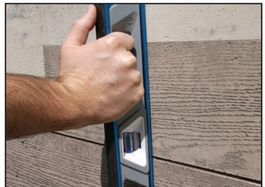
Use a large level to check and maintain an even-face plane over multiple tiles.
