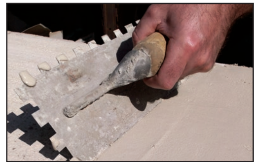
Apply a thin polymer-modified mortar bond coat to the back of the stone.
