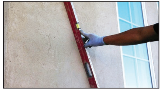
Use a long level or straight edge to confirm your wall is flat.
